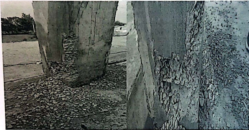
Extremely Poor Quality of RCC Work (RCC Column) GGPS Ali Mohammad Banda (4ACR)
